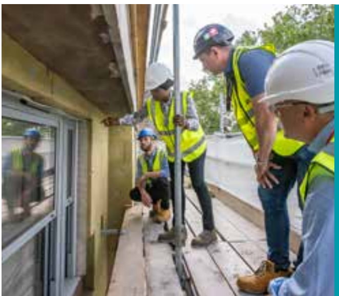
Retrofit project of 66 homes after securing a grant from wave 1 of the SHDF fund.
